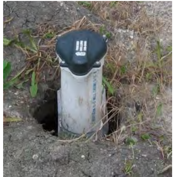
Open annular space outside a well casing which could allow surface water and contamination to enter the well
