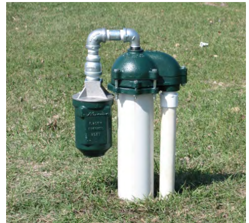
Flood protected well constructed with a watertight cap, snorkel well cap vent and cap cable seal
