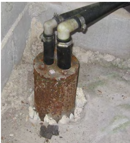
Sanitary well seal on a drilled well
