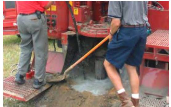
Placement of a surface seal using slurry grout (Photo credit – National Driller, August 2012)
