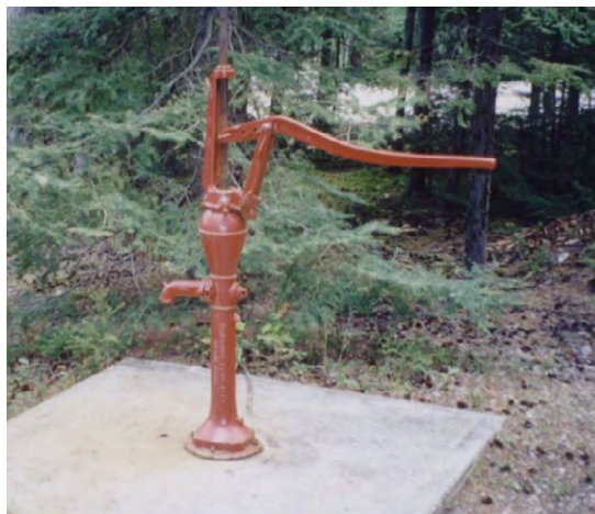
Hand pump with a concrete splash pad
