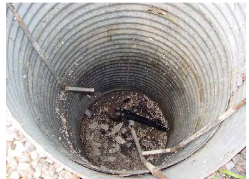
Well located inside of a well pit
