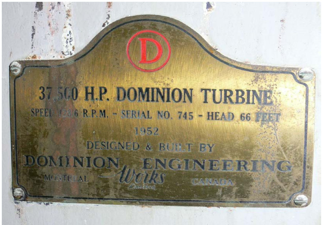
Figure 16 Unit No. 6 Nameplate Original, 1952
