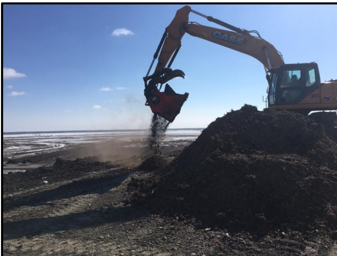
Photograph 3: The blended feedstocks receive a final pass through the hammer mill implement to finish the fabricated soil (February, 2017).
