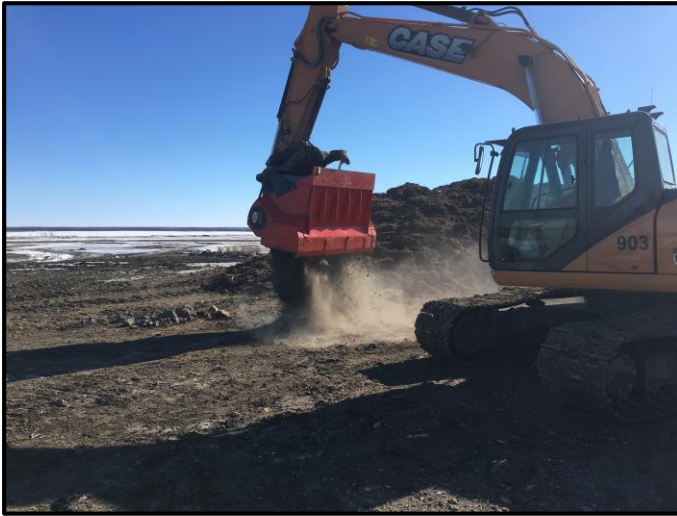
Photograph 1: An excavator fitted with a hammer mill implement grinds frozen clay to a consistency suitable for soil mixing (February, 2017).
