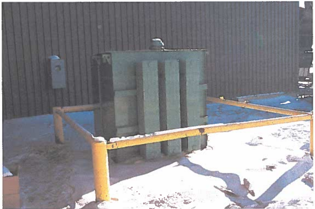
P.10 Transformer Outside Manufacturing Plant
