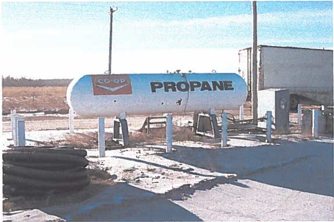
P.01 Propane Storage Tank
