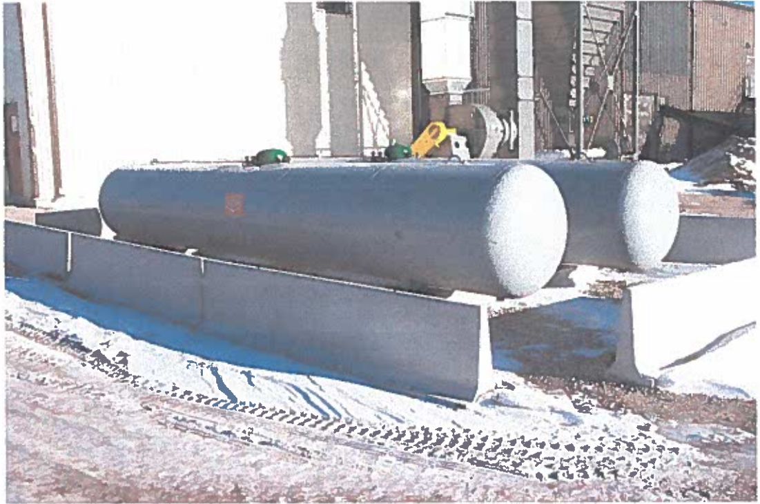
P.09 Second Propane Storage Area
