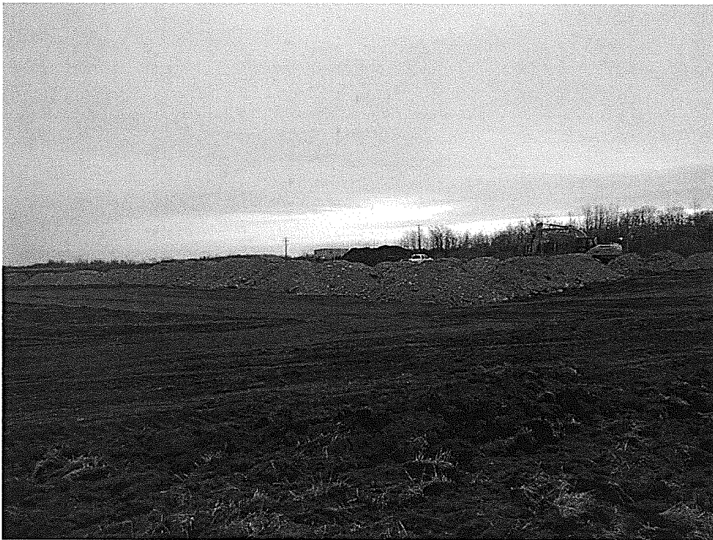
Photo 1 - General view of the project site, with stockpiled pitrun granular fill material
