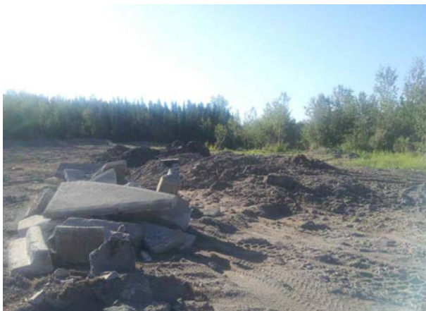
Figure 3.3: Concrete debris at the WWTP Site
