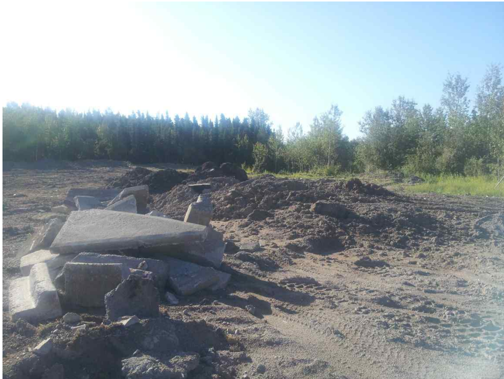
Photo 1 - Concrete debris on the WWTP project site
