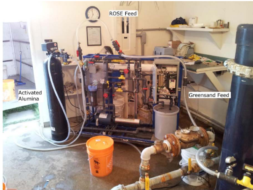
Figure 2: Treatment Process Equipment
