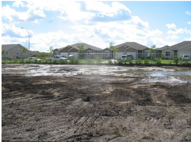
Photograph 13 ↑ Looking west towards Giesbrecht Street and location of the proposed new paver plant (08/01/13).
