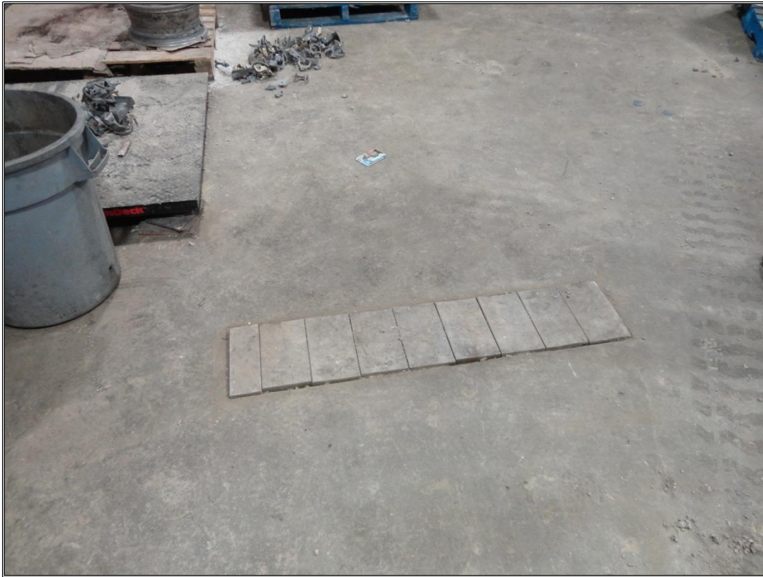
Figure 11: Closer view of the sump pit inside the non-ferrous warehouse. This is a closed pit and is bailed periodically. This sump pit does not drain, nor does it discharge into any water source. In other words, this sump pit is fully contained. In the event of a spillage, the pit can be simply baled and acids would not be discharged into the environment.
