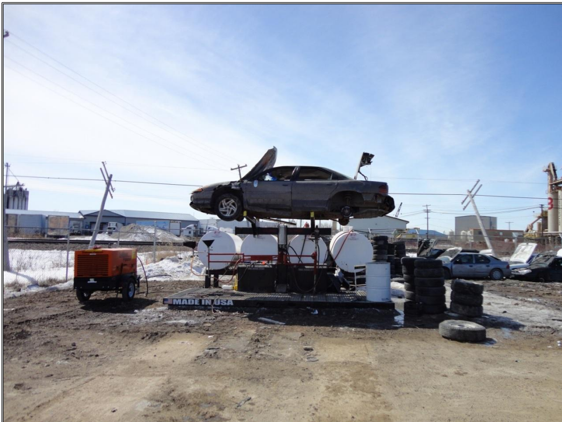
Figure 6: SEDA drain tower and fluid extraction system located near the west perimeter of the site. Waste fluids are stored in the double-walled tanks behind the system.
