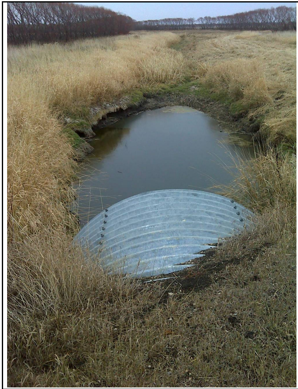
Photo 10: View facing southeast (downstream) of First Creek near the crossing location on the east side of Boivin Road, October 29, 2012. There was standing water in a shallow (<10 cm) pool below the culvert, but otherwise the channel was dry at the time of the field survey.
