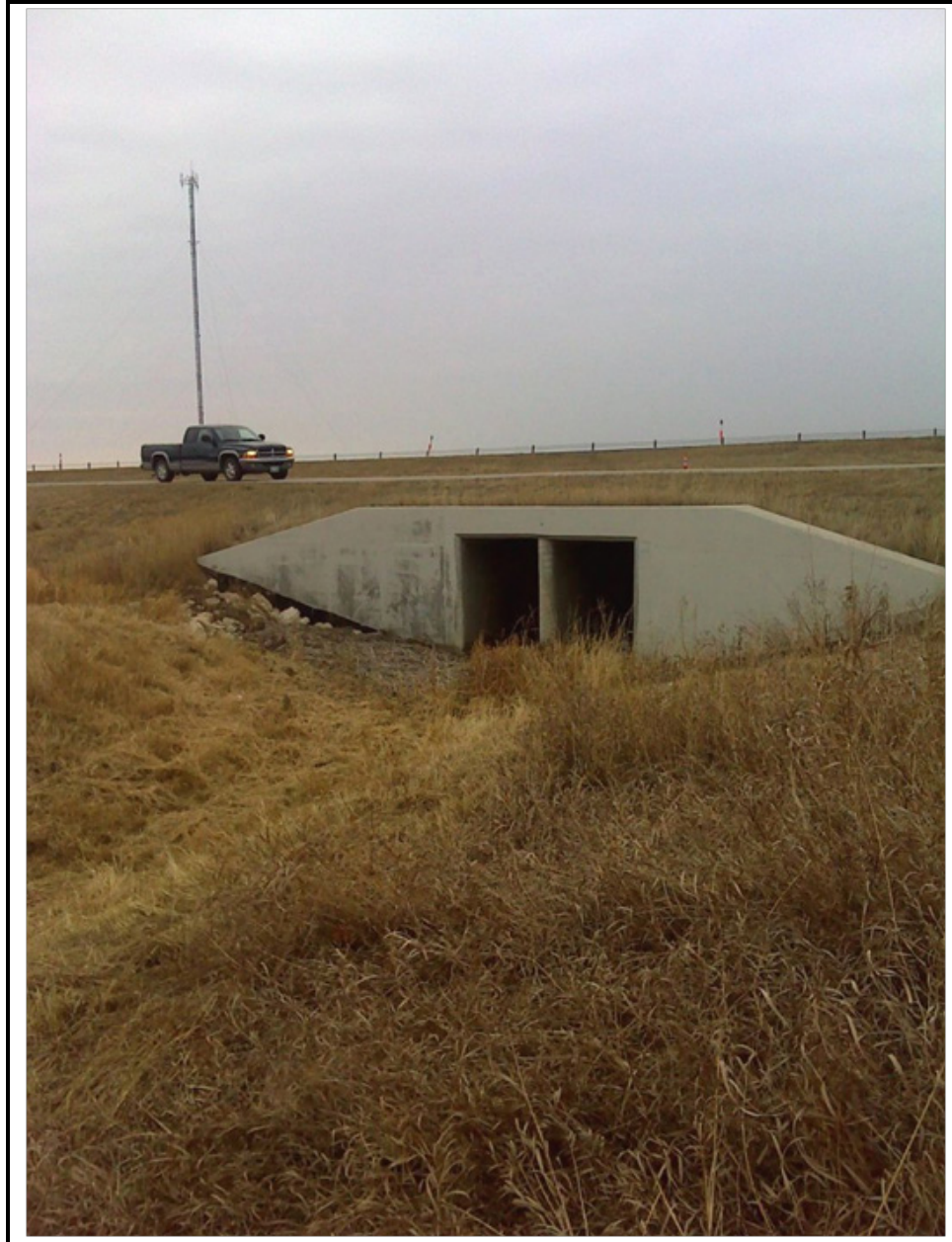
Photo 7: View facing southeast (downstream) of Third Creek near the crossing location on the north side of PTH1 adjacent to the PTH1 service road, October 29, 2012. The channel was dry at the time of the field survey.
