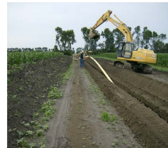
Trenching being undertaken for a past gas pipeline project by Manitoba Hydro
