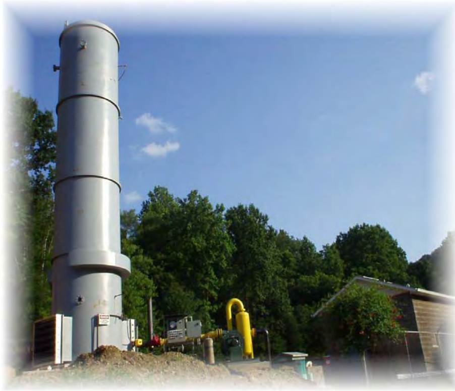
Photo 1-9: Typical landfill-gas recovery system
