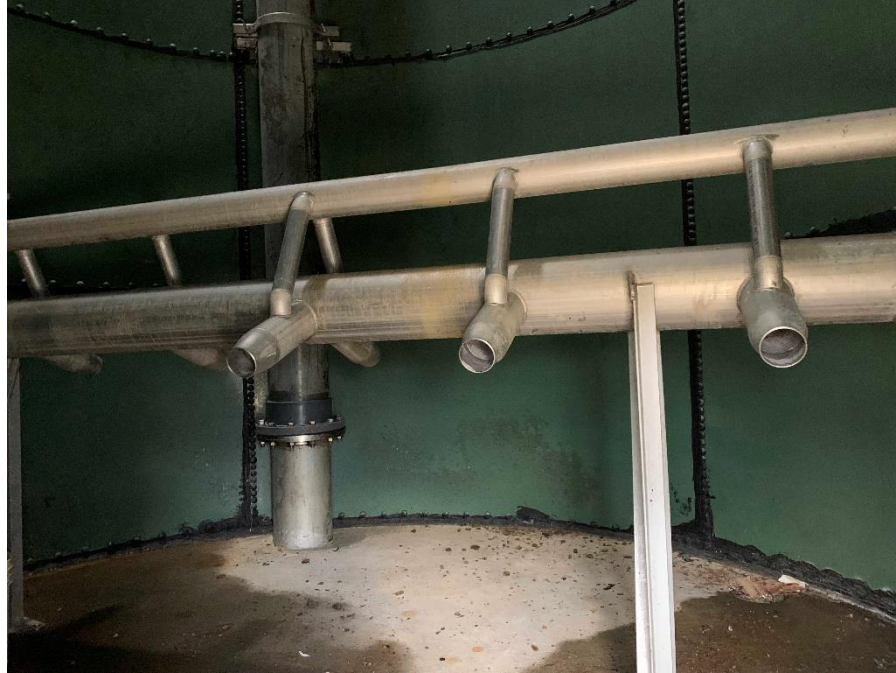
Figure 1-3: Jet Aeration/Mixing System Inside the Stripping Tank
