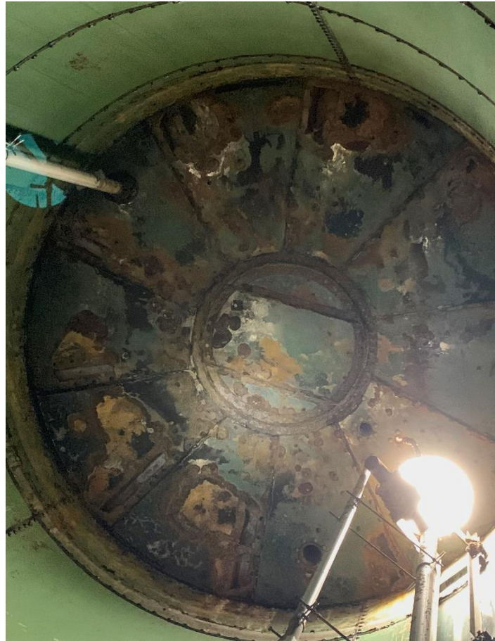
Figure 1-4: Roof Corrosion of the Existing Stripping Tank
