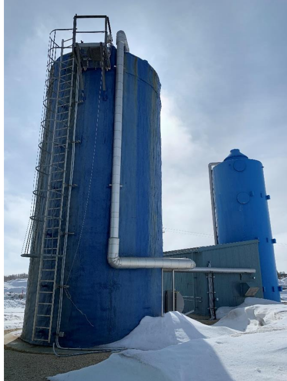
Figure 1-2: Hydrogen Sulphide Stripping Tank
