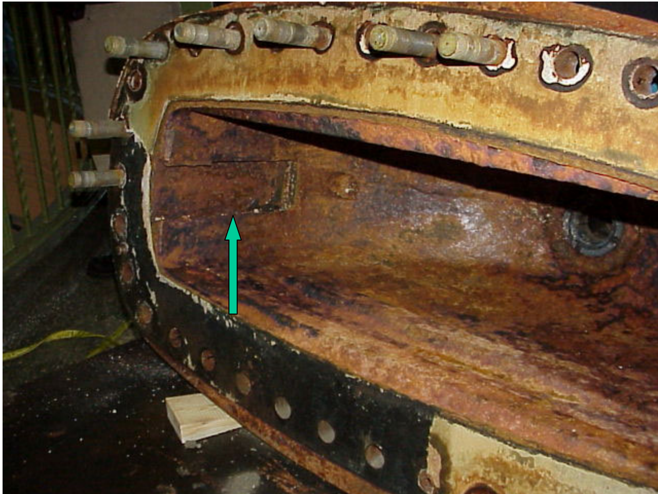
Interior view of valve bonnet showing location from where valve guide bar is missing.
