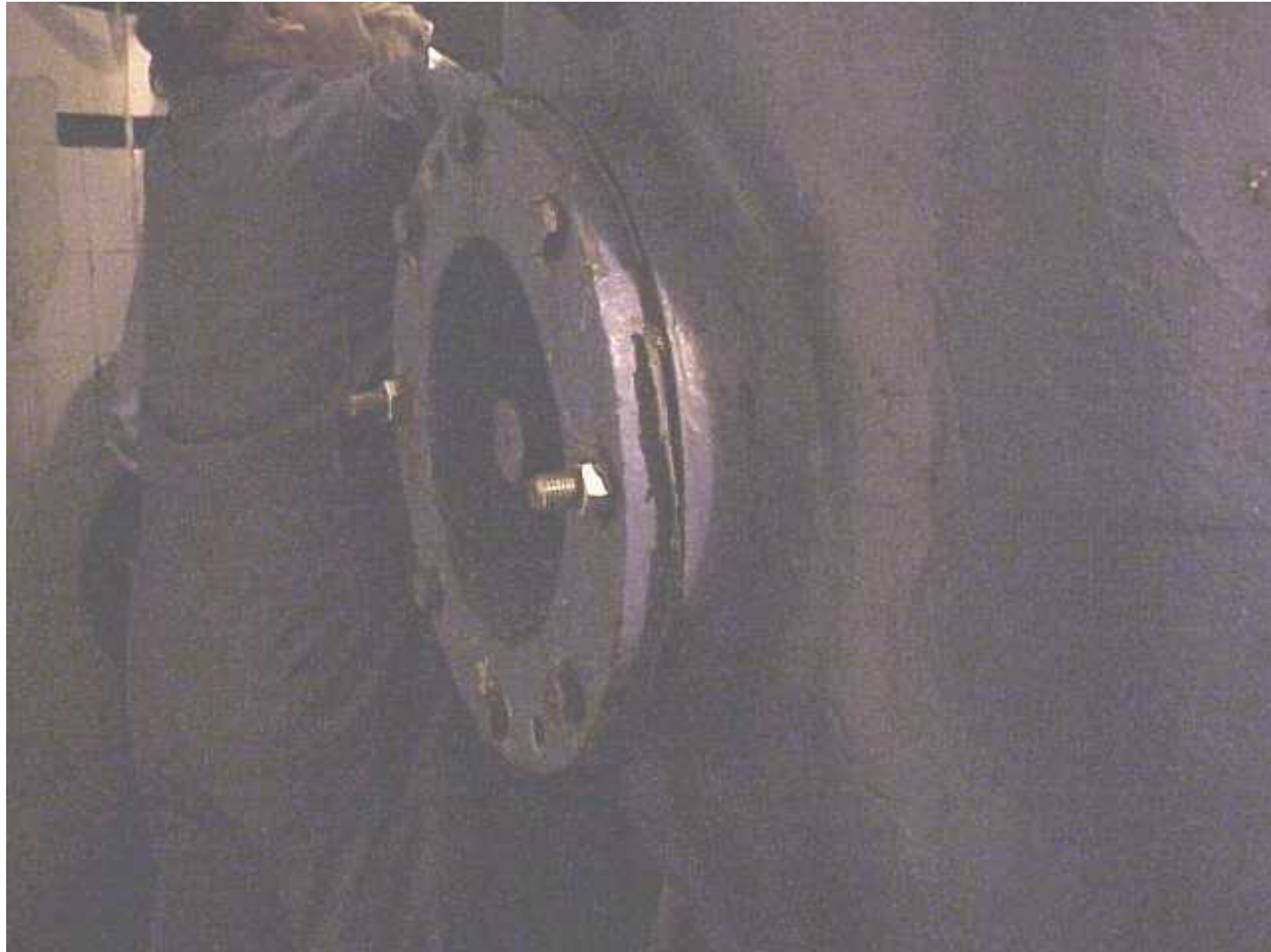
Inspection plate on side of pump MP5
