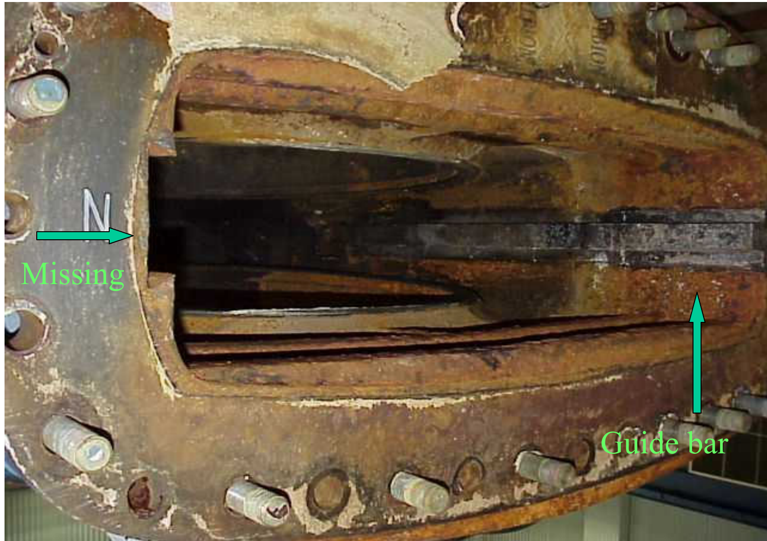
Lower portion of suction valve - guide in place on right side and missing on left side as show by arrows
