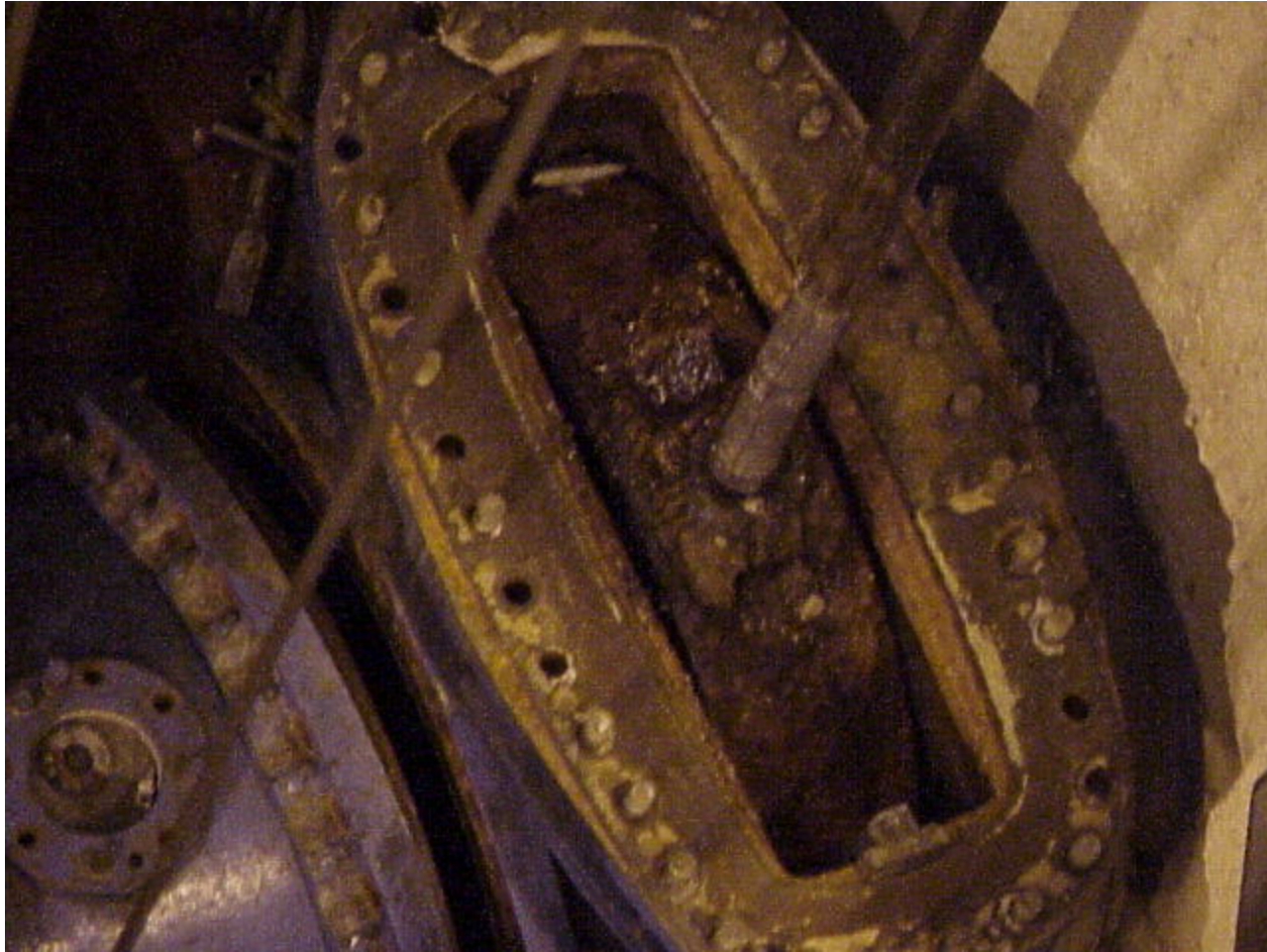
Top view of valve plate and valve stem. Valve had been blocked by a diver to prevent the altering of the location of the valve plate during the dismantling of the valve. The valve could not be removed without partial disassembly
