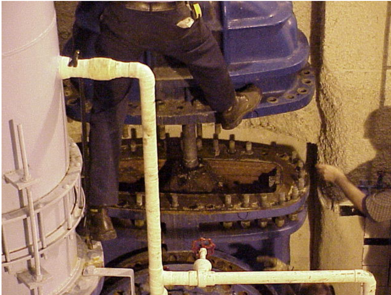
Removal of the valve bonnet - photo shows location of valve plate and attached valve stem.
