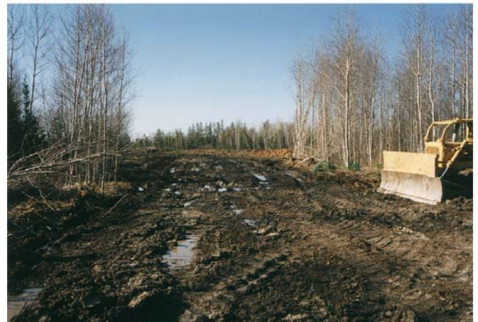
Lack of ditching for surface water run off in this Class III B Road will limit its usefulness.
