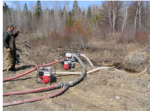
Good example of the Dam and Pump Technique where the sediment is contained and water is pumped allowing for a dry installation
