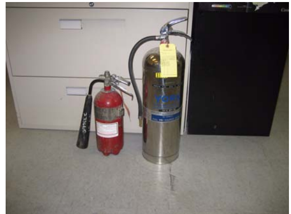
Inspect fire extinguishers in your camp and on-site equipment each month
