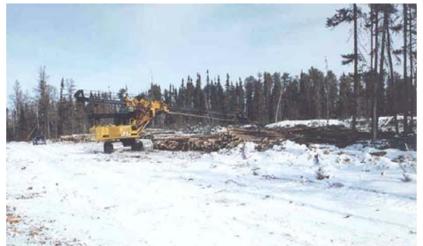
Example of light impact landing – no bulldozing and efficient use of road right of way
