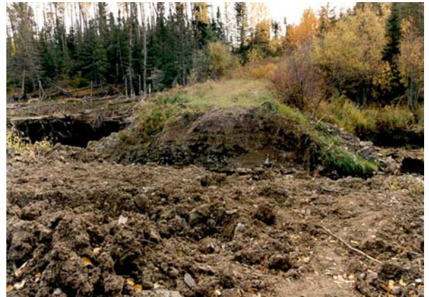
Culvert removal with improper sloping
