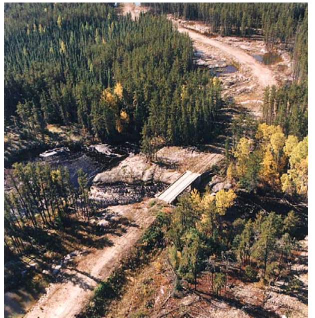
Reduce right of way clearing width near water crossings to minimize the potential of soil erosion
