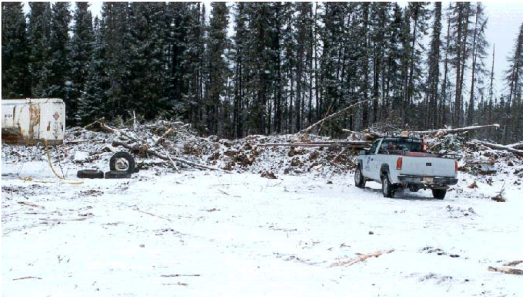
Unacceptable bulldozed windrow of debris containing usable trees
