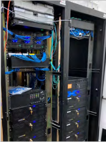
New Video Surveillance System Head-end Equipment at the MLB
