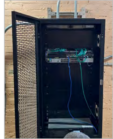
New Video Surveillance Network Equipment at the Government House Building
