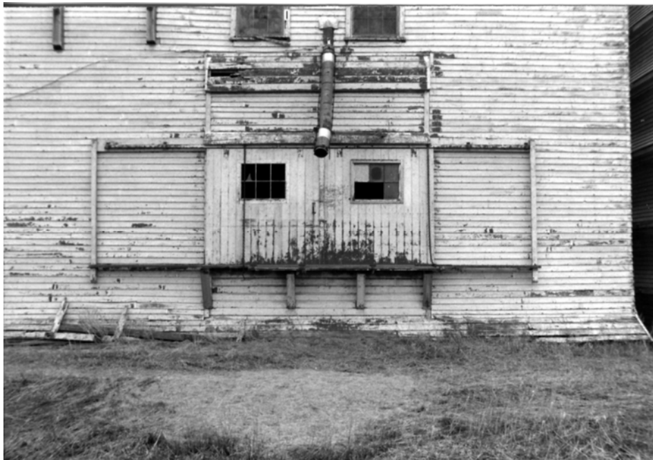
Two views of a car-spout. Some elevators had the car-spout located entirely on the exterior of the building, while in other cases only the bottom end of the duct was exposed. (top: La Rivière 282.L.2; bottom: Lenore 291.L.1)
